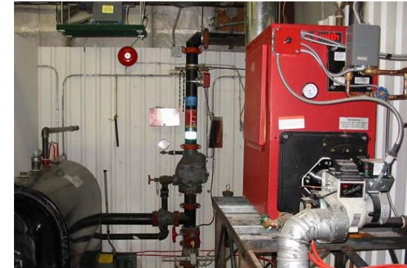
Green Technologies' boiler running 100% biodiesel
