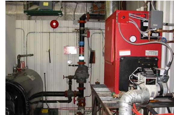
Green Technologies' boiler running 100% biodiesel
